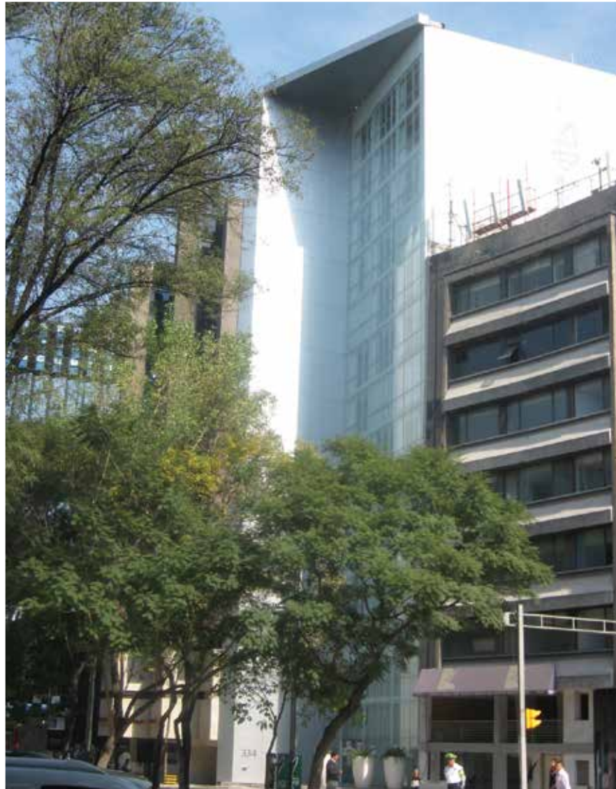
Three Capstone C65 Microturbines provide electricity and heating at this prominent hotel in Mexico City.
