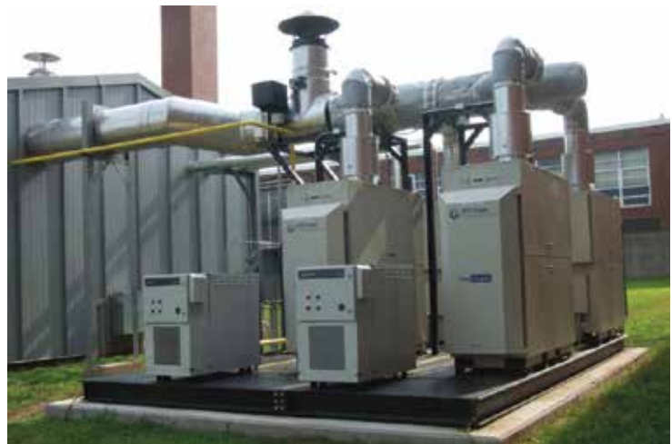
A PureComfort® 240M solution featuring four 60kW Capstone microturbines provide cooling, heating, and onsite power to East Hartford High School in Connecticut.
