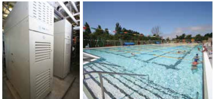
Two Capstone microturbines help control power costs at this recreation center in Santa Cruz.
