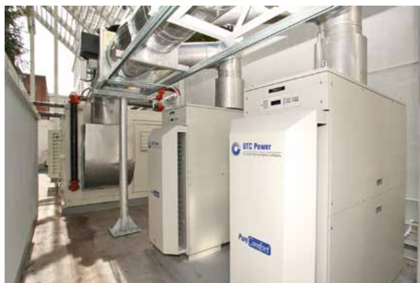
Four 60kW Capstone microturbines provide cooling, heating, and power to the prestigious Ritz-Carlton hotel in San Francisco.
