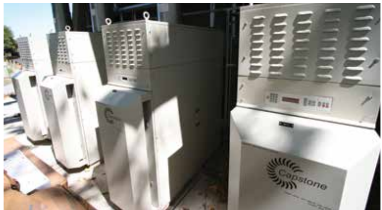
The pool at Foothill College is heated by four C60kW Capstone ICHP microturbines.
